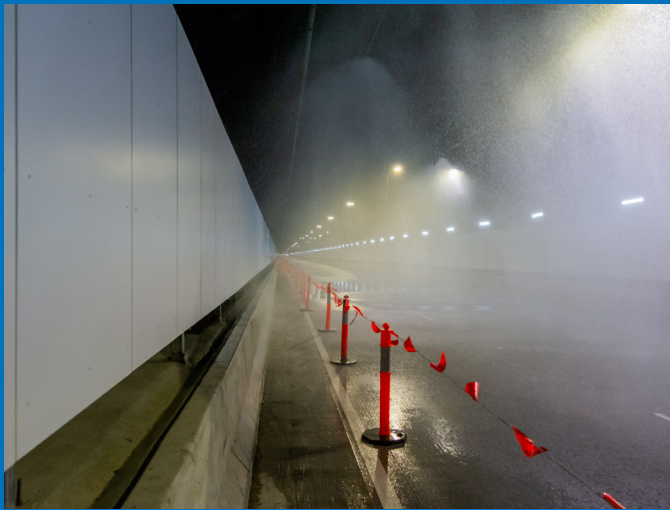
Testing of deluge system in 'New M4' Tunnels
